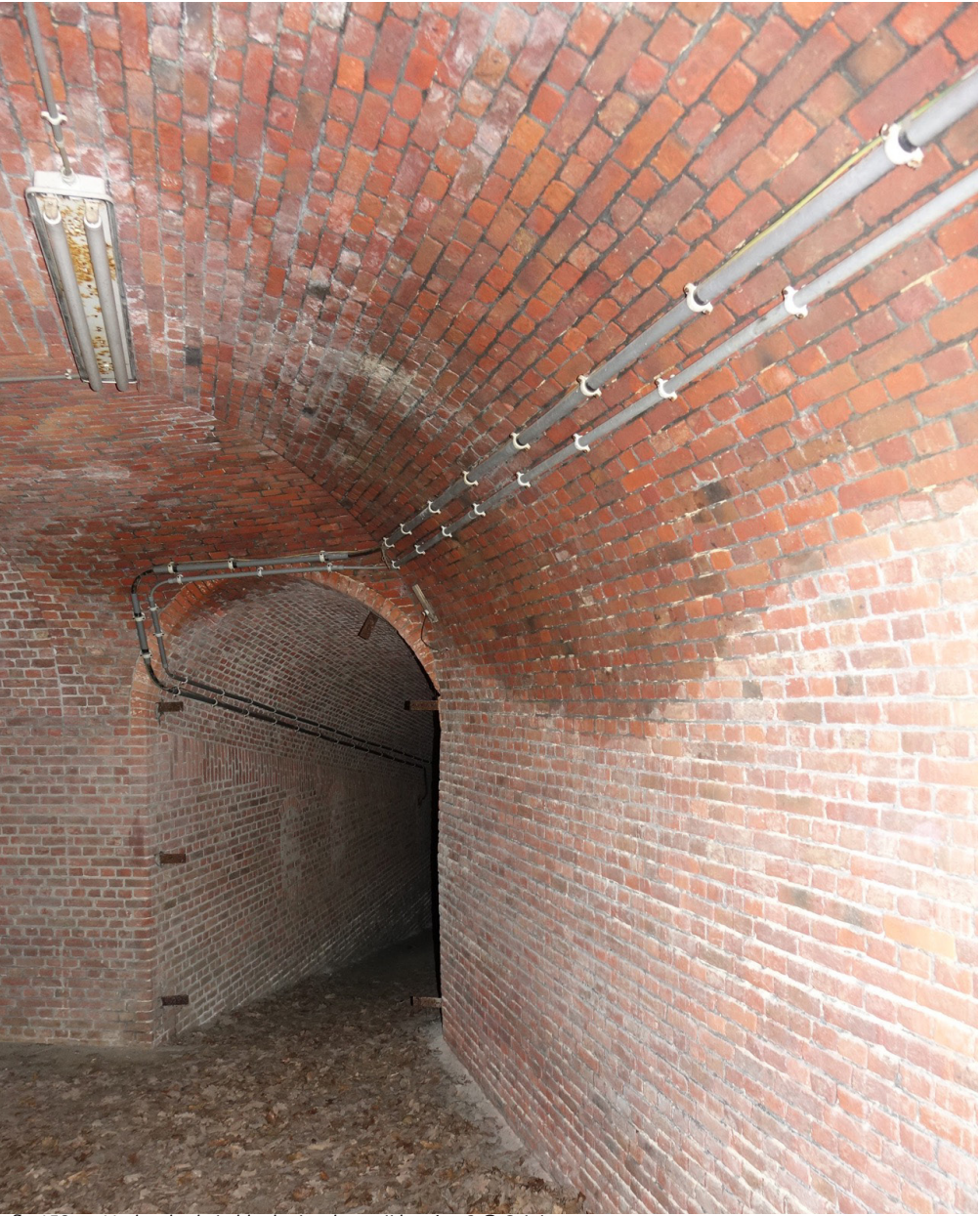
afb. 158: Vochtschade in blankeringsbatterij bastion 3 © Origin
