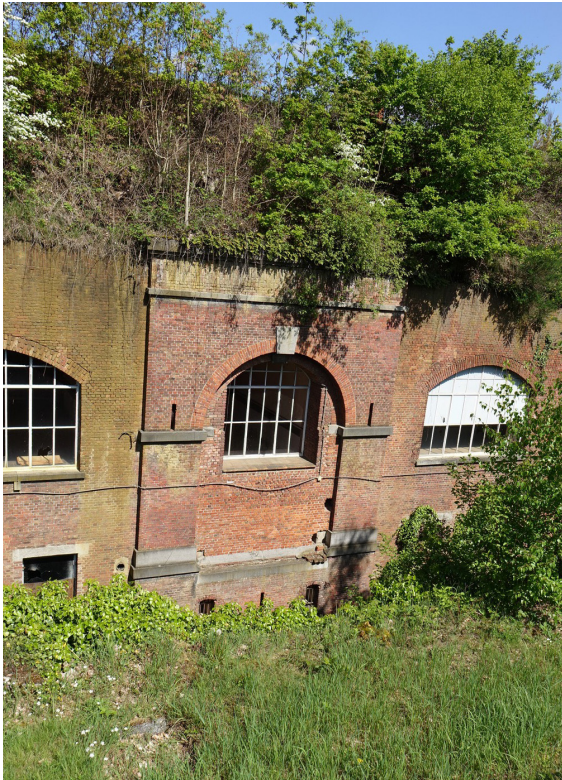
afb. 113: Centrale poterne front 2-3 © Origin
